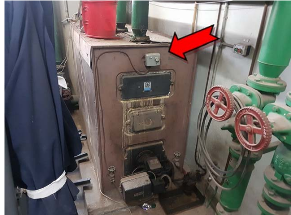
Photo 8. Interior, ground floor, southern store, throughout, boiler internal – asbestos containing gaskets.
