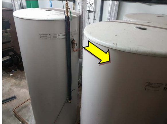
Photo 14. Interior, ground floor, southern store, hot water heaters – suspected SMF-containing internal insulation.
