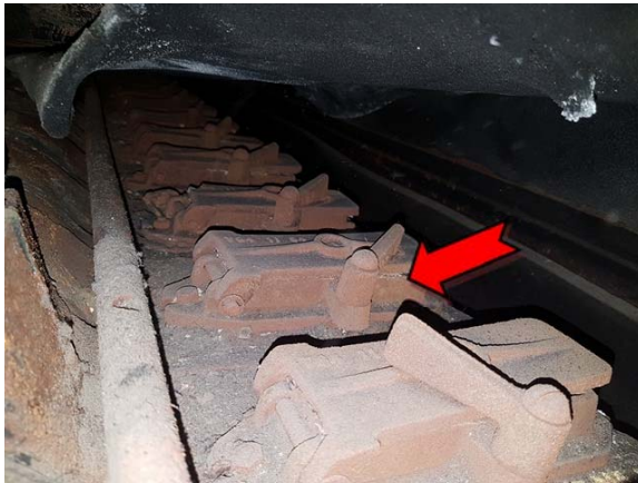
Photo 9. Interior, ground floor, southern store, throughout, boiler internal – asbestos containing gaskets.
