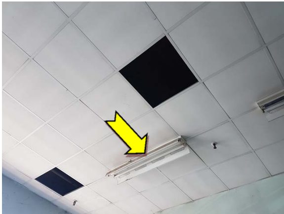
Photo 15. Interior, throughout, fluorescent light fittings – suspected PCB-containing capacitors.
