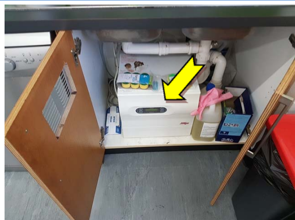
Photo 12. Interior, level 1, staff room, hot water heater – suspected SMF-containing internal insulation.
