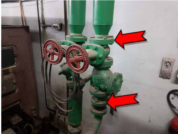
Photo 7. Interior, ground floor, southern store, throughout, pipework – asbestos containing gaskets.
