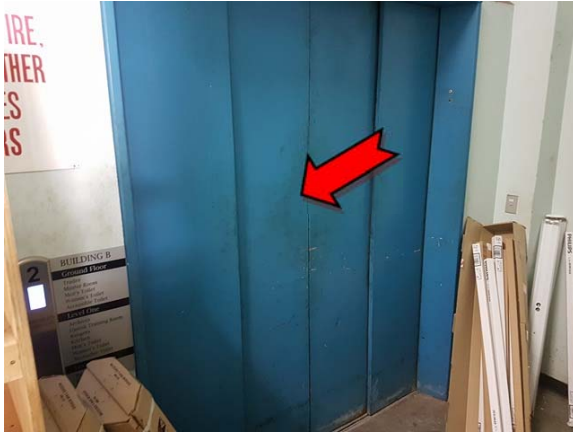
Photo 1. Interior, level 2, lift door – suspected asbestos containing door core.
