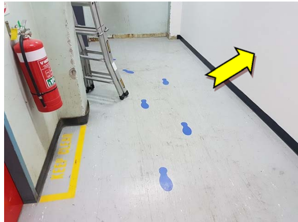
Photo 16. Interior, level 2, throughout, walls – suspected lead upper coloured blue paint system.
