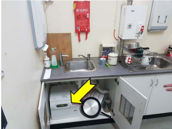
Photo 13. Interior, ground level, lunch room, hot water heater – suspected SMF-containing internal insulation.
