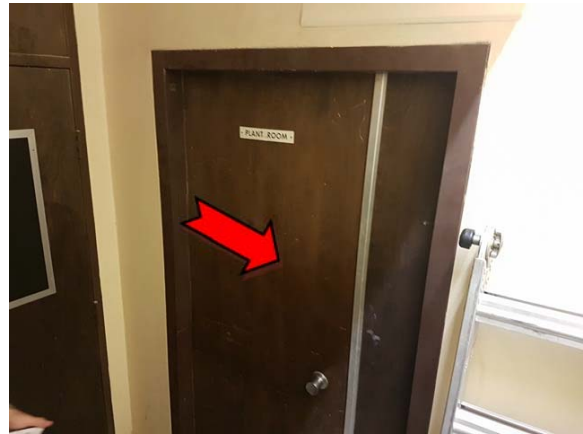
Photo 4. Interior, level 1, plant room, entrance door – asbestos-containing core.
