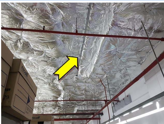
Photo 11. Interior, level 1, archives room, ceiling – suspected SMF containing sarking insulation.
