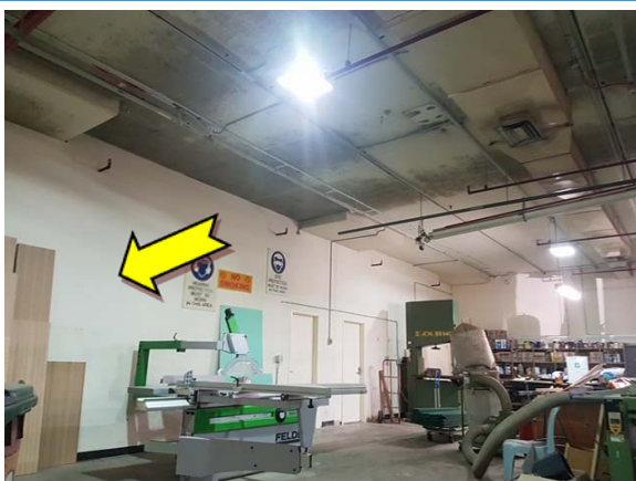
Photo 17. Interior, ground level, throughout, walls – suspected lead upper coloured white and cream paint systems.
