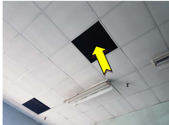
Photo 10. Interior, level 2, store, ceiling space – suspected SMF containing sarking.
